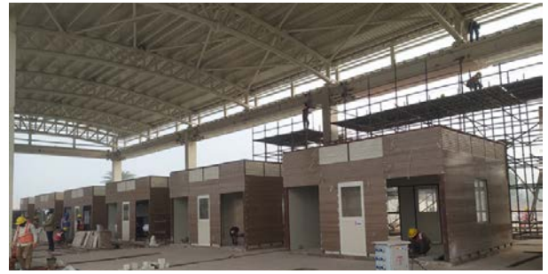
Figure: Prefabricated Porta Cabins installed in a PEB Shed structure for Security scanning at the entry of a complex
