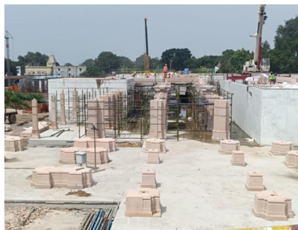
Figure: Typical courses of each columns are produced and assembled at site
