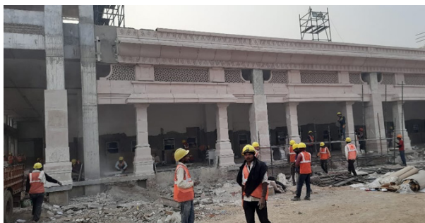
Figure: Modular Cladding prefabricated in factory and installed on RCC columnar structure
